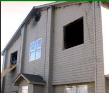
Building burned in the fire
